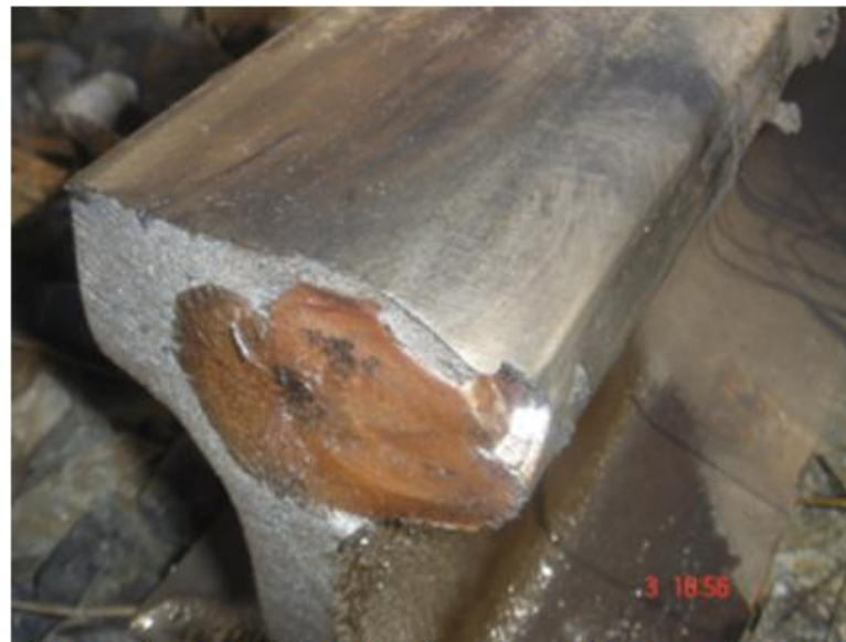
Figure 1b. DSS defect that has turned into a transverse defect and broken the rail under traffic.
